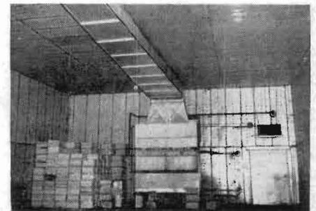
The only equipment in the room is an evaporator with blower and duct work and the caustic soda spray chamber.
