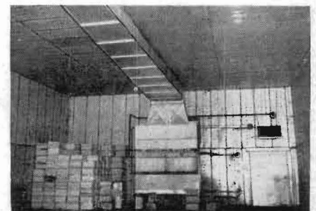
The only equipment in the room is an evaporator with blower and duct work and the caustic soda spray chamber.
