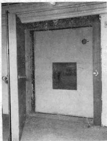
A sealed door with an observation window is important.
