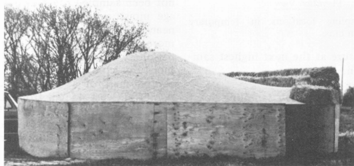
Figure 2. Wind damage to open-topped temporary grain bin (bin no. 3, Table I).
