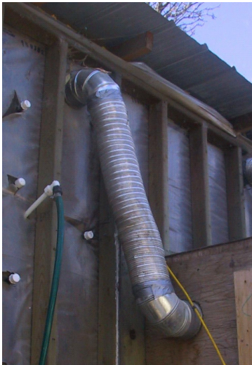
Fig. 4. Flexible aluminum duct attached to exhaust supply (bottom) and inflatable bladder (top). Air from the exhaust supply pressurized the bladder.
