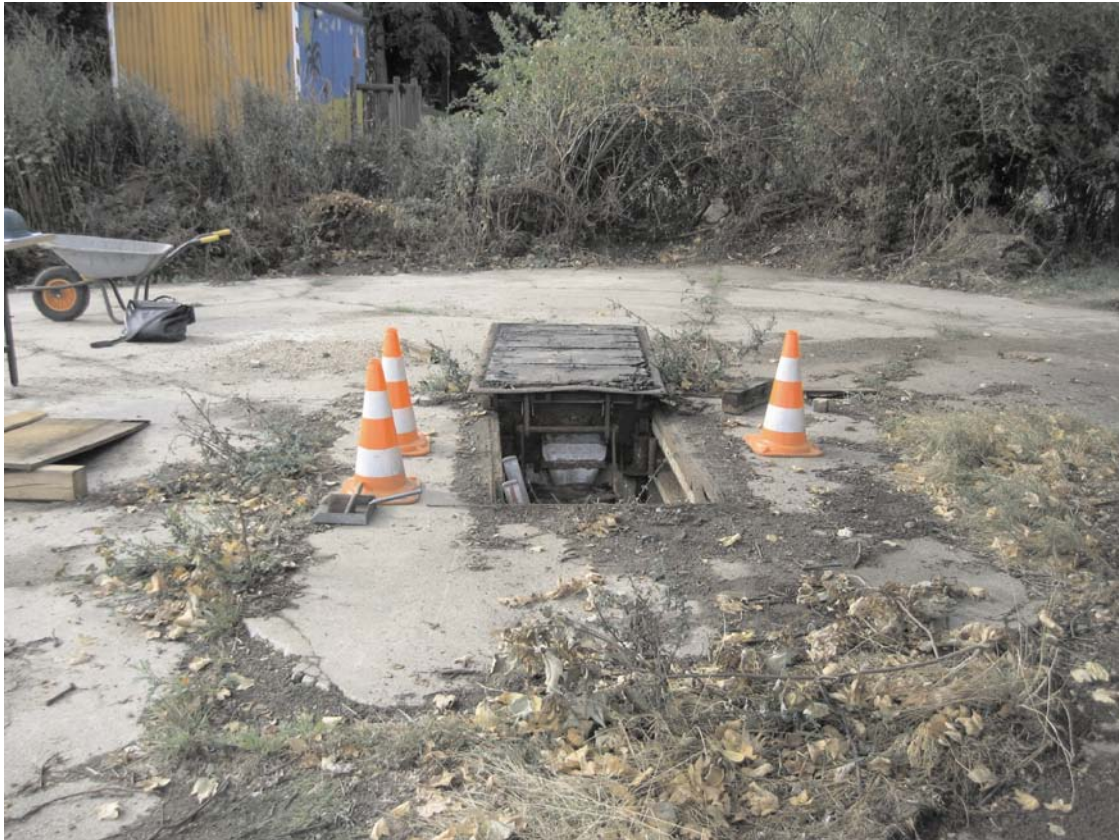
Figure 6. View of a 72 years old container made of reinforced concrete.
