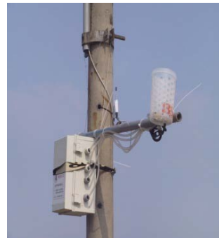
Fig. 3. Universal dust sample collector installed at 3m height.
