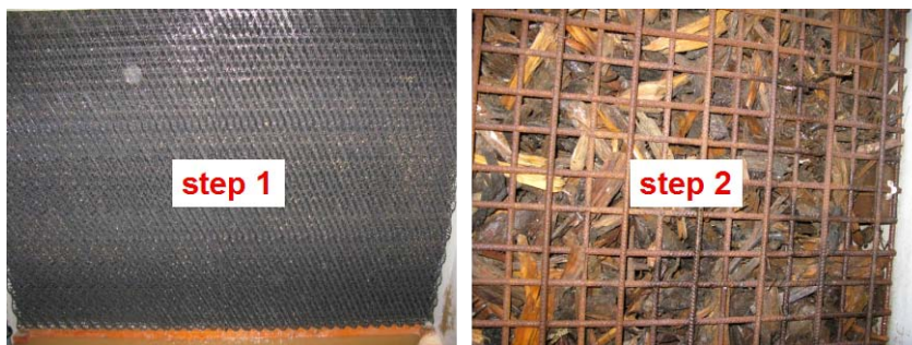
Figure 3. ScanAirclean A/S chemical air scrubber in combination with a biofilter consisting of 60 cm crushed tree roots.
