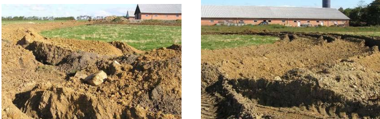
Figure A2. 8 km of PE tubes were placed 4.0 m deep in an adjacent field using a chain excavator.
