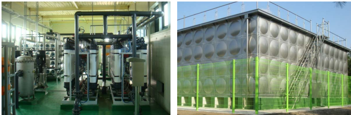
Figure 8. View of wastewater reuse system (left) and storage tank (1,000 m 3 ) of reclaimed wastewater (right)
